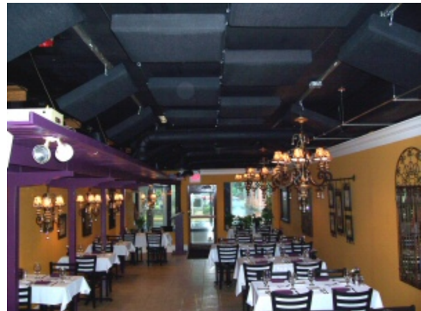
Acoustic Panels mounted on the restaurant ceiling
